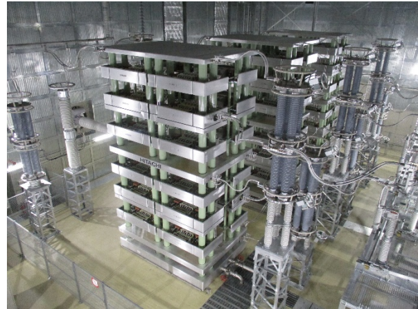
A valve hall equipped with a line commutate converter HVDC (AC/DC converter)
