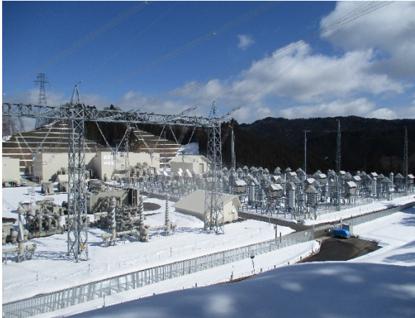
Hida Converter Station of Chubu Electric Power Grid Co., Inc.
