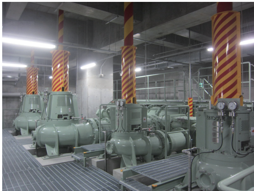
2 Zenigamecho Pumping Station pump room
