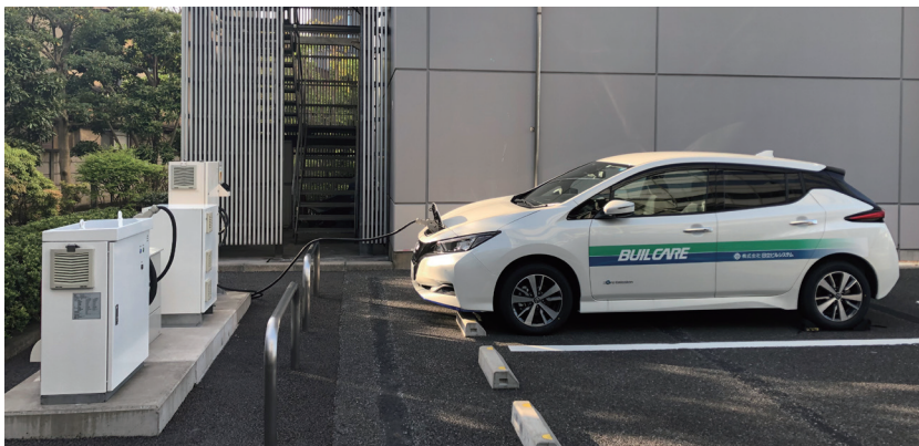
2 V2X system utilizing a hybrid PCS introduced at the Kameari General Center
