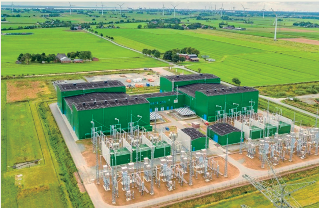
NordLink, a \pm 525 -kV/1,400-MW and about 600-km HVDC link that connects Norway and Germany
