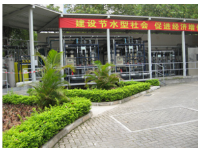
Wastewater recycling system (Shenzhen Waterworks Model Project, 2007)
