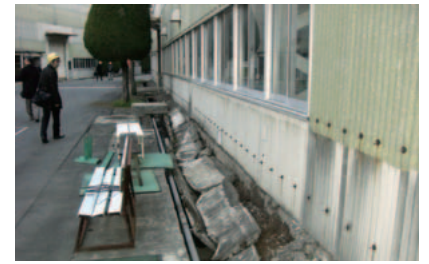
Hitachi Works after the disaster. Many Group factories were damaged.
