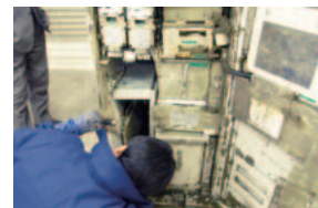
The tsunami caused major damage to 20 ATMs. Engineers tackled tasks such as repairing ATMs with case damage.
