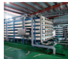
Hitachi Plant Technologies' Reverse osmosis desalination system
