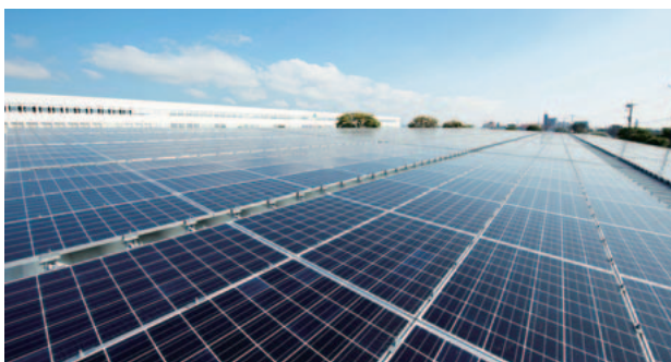
Photovoltaic system installed at Omika Works
